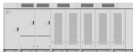
NBSK - LV station
